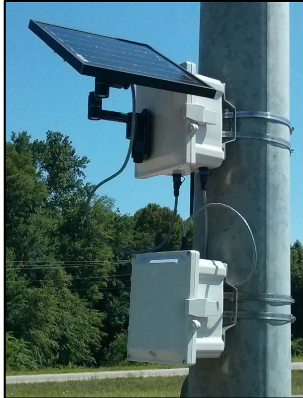
Figure 3: Example Bluetooth Sensor Installation
