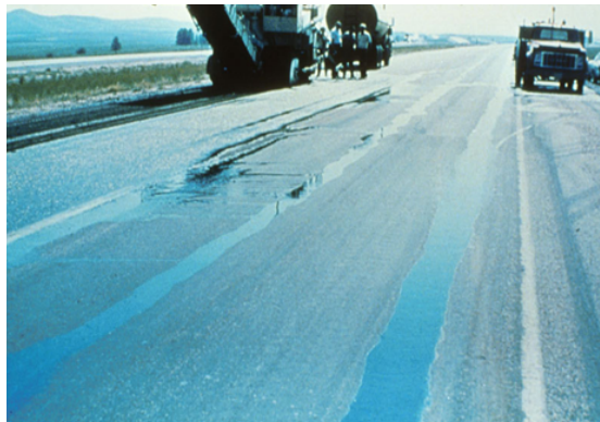
Figure 7: Examples of rutting distress in asphalt pavement.
